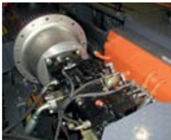
E-drive and main pumps
